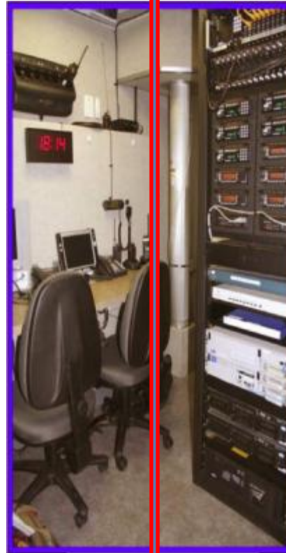
Control Room "Interoperability" Mission Management Operator, Equipment Racks and shelves for Interoperability (30') mast.
